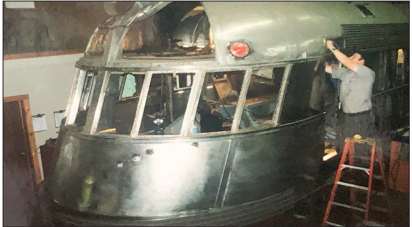
A crew member at the Concord and Claremont Railroad is shown working on the Flying Yankee in August 2002 after it was moved to Claremont in 1997 from Glen before finding a home at the Hobo Railroad in Lincoln in 2005. (TOM EASTMAN/MOUNTAIN EAR PHOTO)
